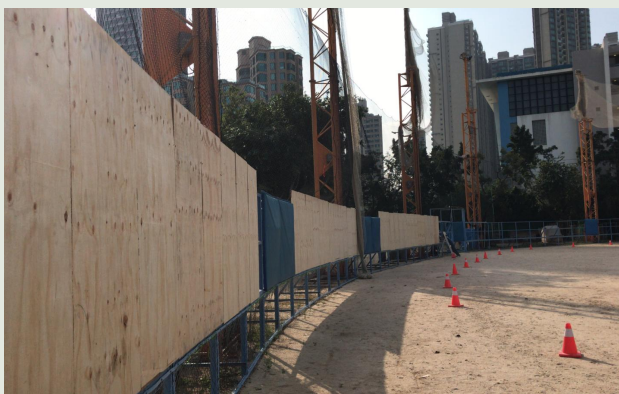
上：球場外野臨時設施 Above：Temporary remedies at the outfield
